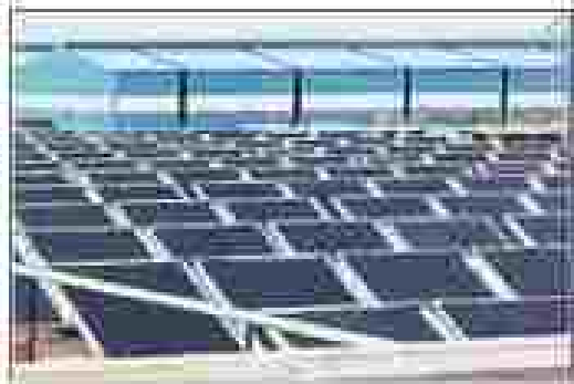
Fig 3.17: Solar Panels to trap solar energy
